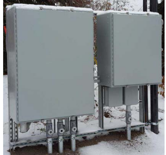
HIGH VOLTAGE and LOW VOLTAGE PANEL
